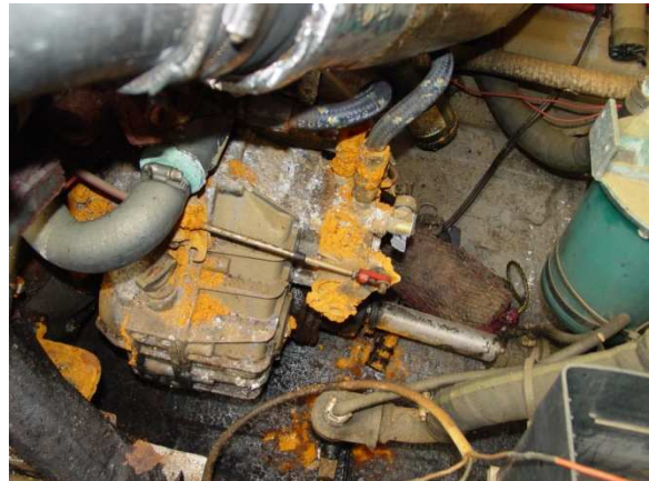
Photo 5: Example of engine corrosion
