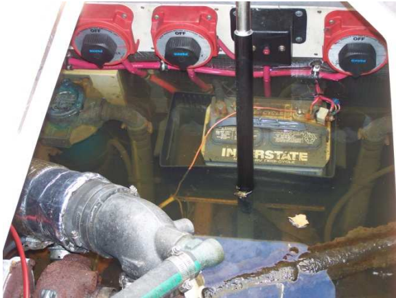
Photo 1: Flooded engine compartment
